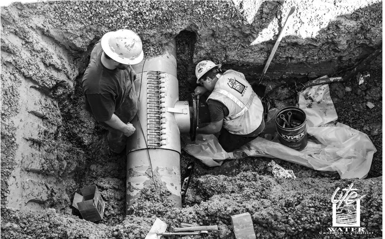
Above Photo by Joe Burtard - Utility Maintenance Workers, Cody Walker (Left) and Dusty Kriegshauser (Right) performing live tap on a 12-inch line on Horizon Drive.
